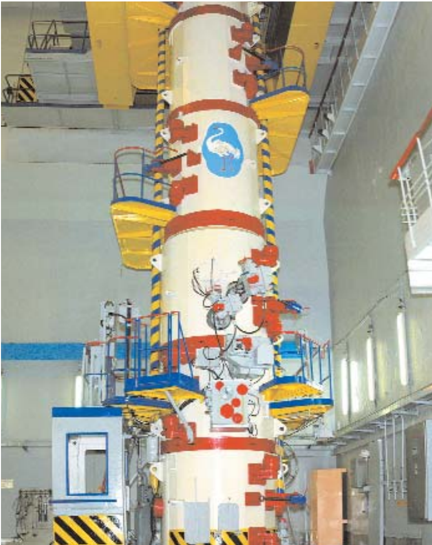
A special refueling machine supplies fresh fuel and removes fuel waste from the operational reactor.
